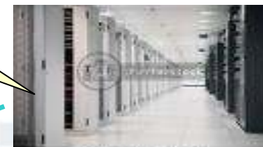
Data centers or server rooms
